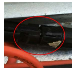
The cable is loose
